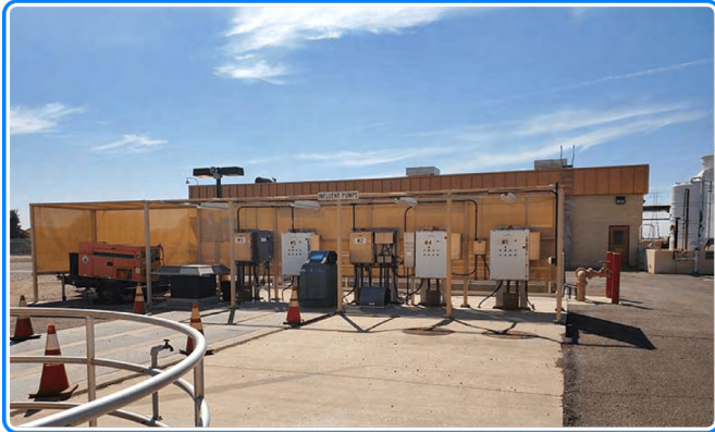
Influent Pump Control Cabinets: Exterior monitoring control cabinets for the influent pump station where wastewater from the city's collection system enters the processing plant and is pumped to the beginning of the treatment process.
