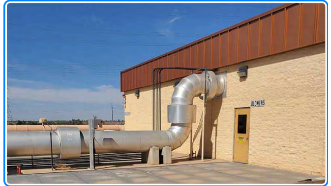
Aeration Basin Air Header: The City of Peoria's Aeration Basin Air Header ensures the wastewater treatment system maintains and aerobic condition and improves the water quality for subsequent usage. This process helps get rid of bad bacteria before water is percolated into the ground water system.
