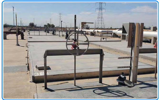
Aeration Basin Flow Control Gate controls the pressure and flow of air for treatment ponds and promotes biochemical oxidation of wastewaters.
