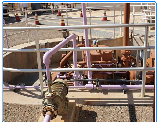
Grit Chamber, grit pump and grit seal water pump: The grit chamber primary catches inorganic solids such as sand, gravel, glass, corn, and soil.
