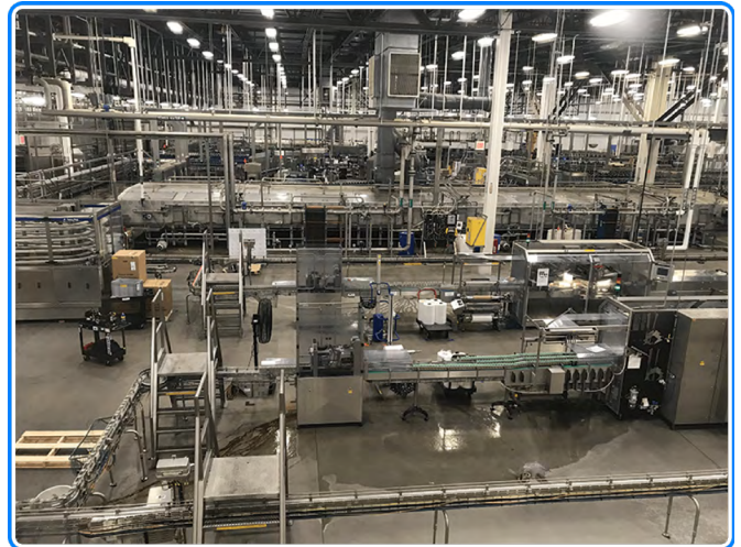
GE iFIX coupled with WIN-911 Advanced remote alarm notification software helps ensure the plant maintains operations 24/7.
