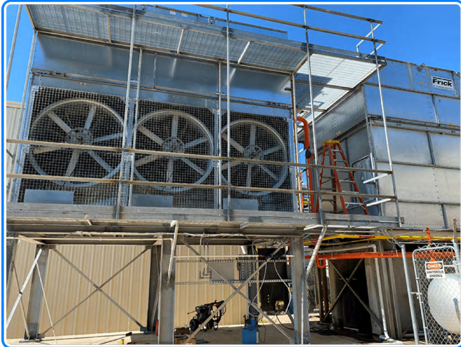
SmartSights WIN-911 software monitors each stage in Night Hawk's sophisticated refrigeration process. This includes the company's state-of-the-art refrigeration system's cooling towers, which remove excess heat and maintain precise temperatures.
