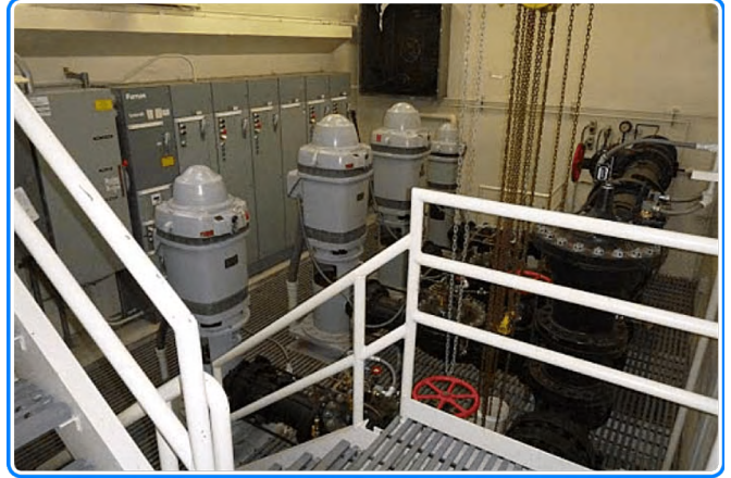
A water inlet station shows water pumps for distributing source water to customers. WIN-911 monitors over 70 of these remote stations for the Bellevue water service.
